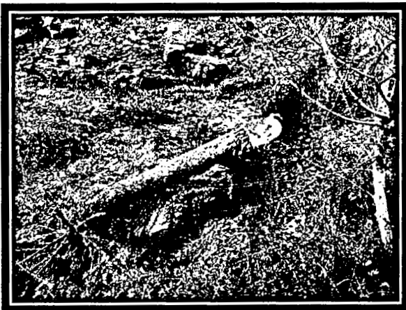
Photo 8: Sewage line break
