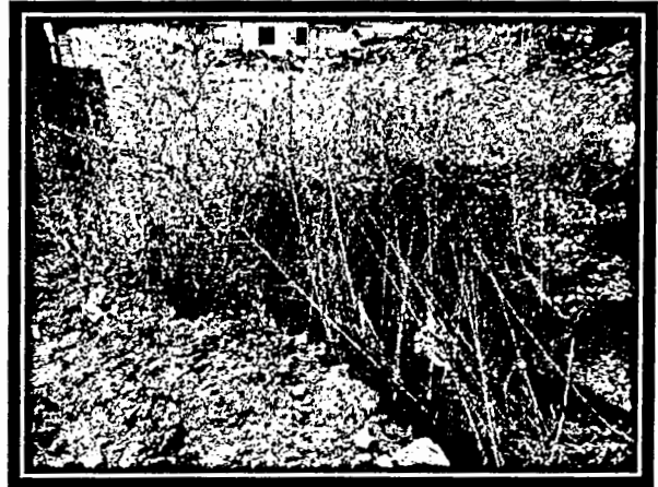
Photo 10: Cesspool from sewage line break
