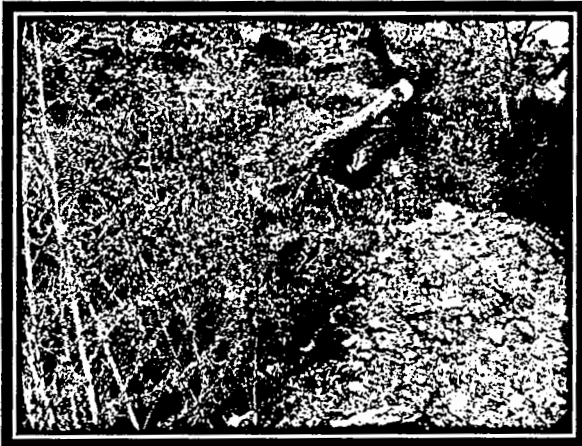
Photo 7: Broken sewage line
